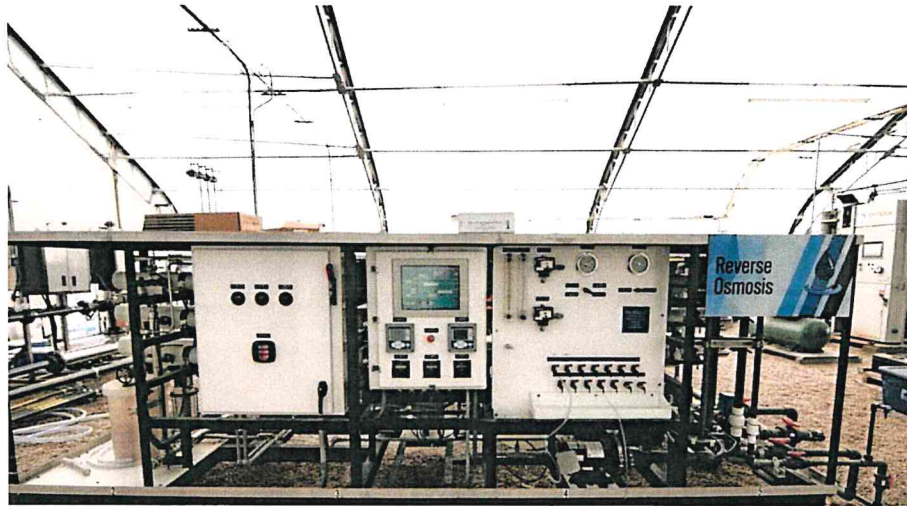
Reverse Osmosis/Membrane Softening/Nanofiltration Pilot
